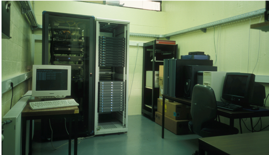
Figure B.2: Picture of the computing farm room. The central rack contains the 24 machines, with the twelve PIII on the top and the twelve dual Xeon on the bottom. On the right we can see the mass storage as well as the software repository.
